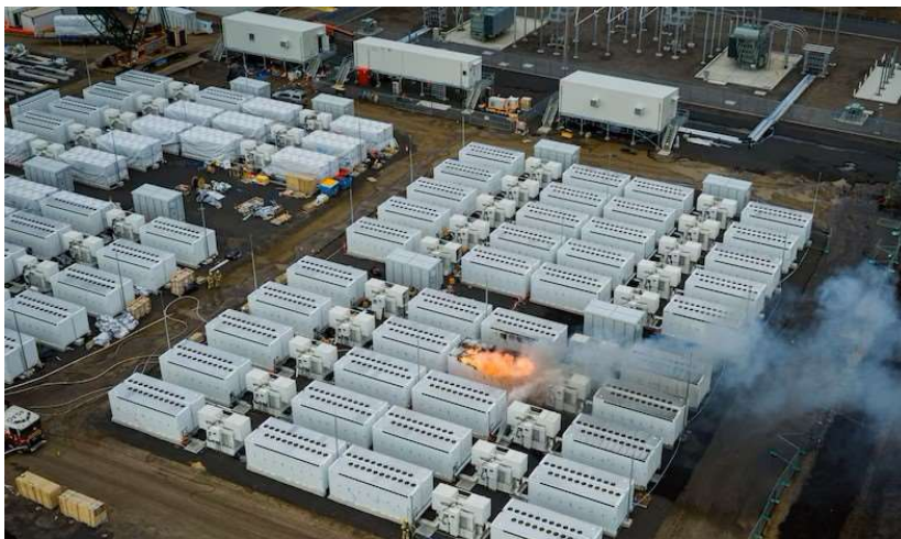
Figure 3 Big Battery Fire (Supplied by FRV Aviation Unit)
