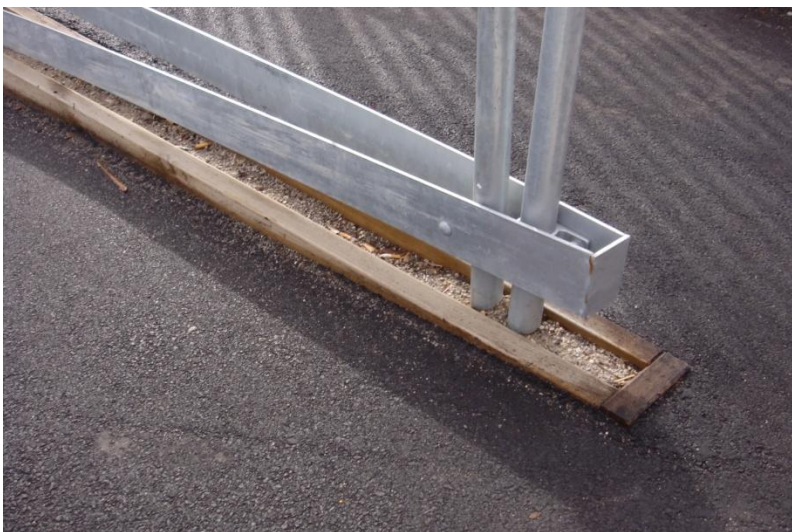
Lack of appropriate kerb rails
