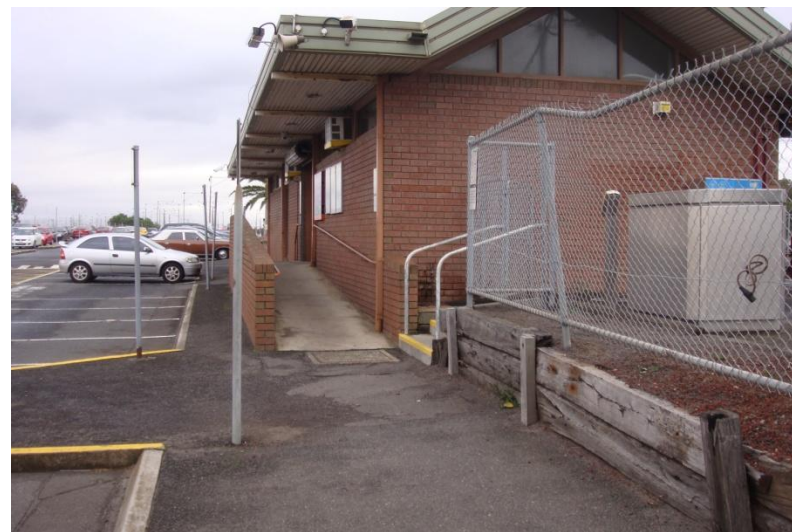
Lack of tactile ground surface indicators
