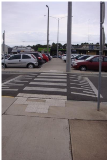
Damaged tactile ground surface indicators
