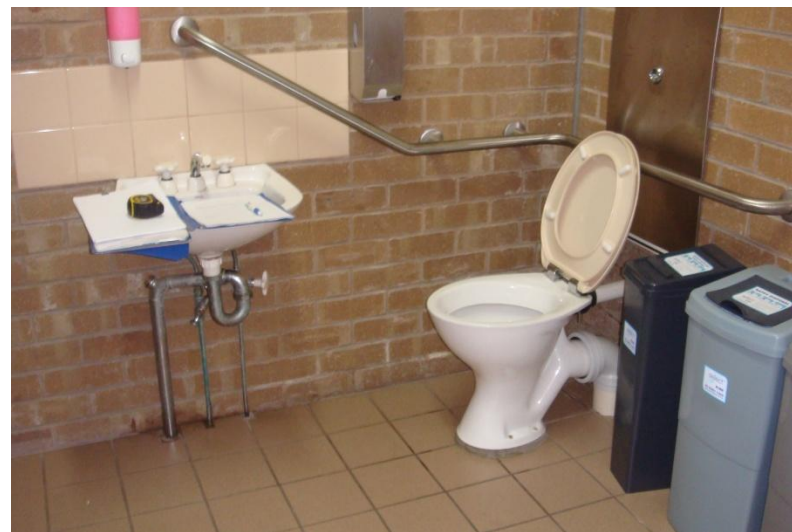
Fixtures and fittings installation inappropriate
