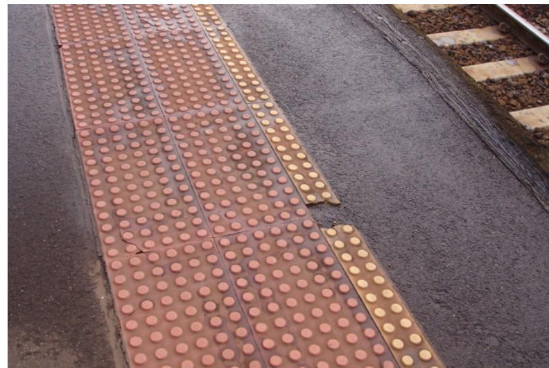
Damaged tactile ground surface indicators
