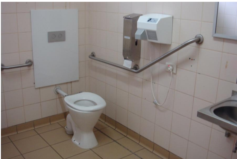
Inappropriate placement of fixtures and fittings
