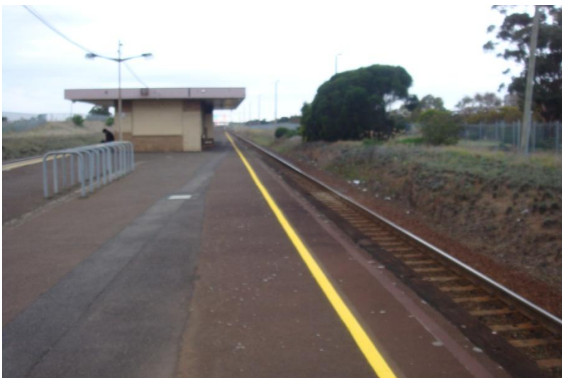
Lack of tactile ground surface indicators
