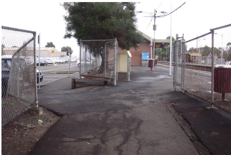
Lack of directional tactile indicators
