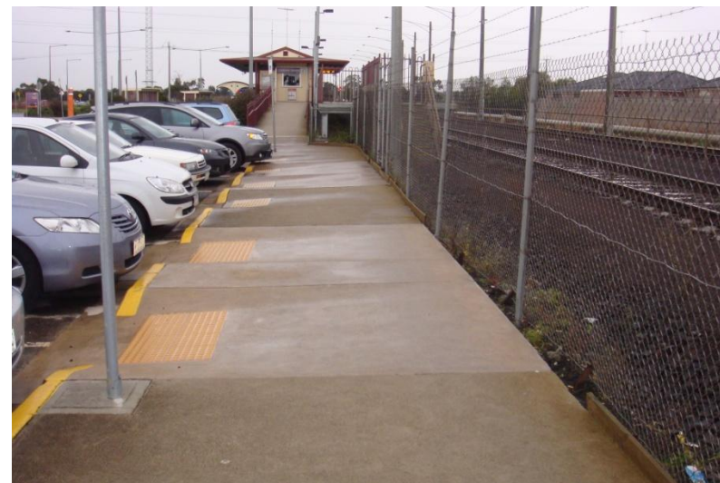
Inappropriate kerb ramps limit access
