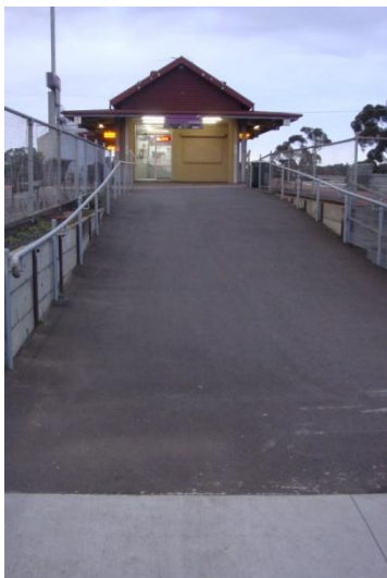
Lack of appropriate gradient and kerb rails
