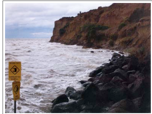
Photo 8 Restricted beach access at high tide
