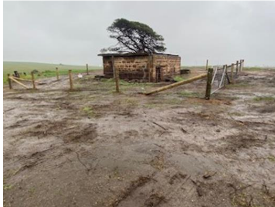
Former Dairy Outbuilding following the removal of the roof and other historic adjoining fabric, 2020. Source: Michael Burge, City of Greater Geelong.
