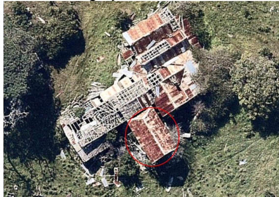
Aerial image, 9 September 2018. The surviving wing of the dairy outbuilding, showing the 'front' hipped roof face is circled. Source: NearMap.
