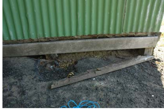
Photo 3.59: Market Offices building, south elevation. Detail of rotted timber base boards.
