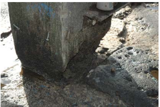
Photo 3.26: Detail of rotted base of timber post.
