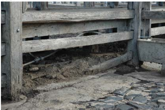
Photo 3.24: Detail of rotted subfloor structure of covered walkway.
