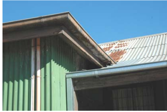
Photo 3.61: Market Offices building, east elevation. Detail of junction of hipped window and main traversing roof. Note the completely rusted gutters on the projecting hipped wing.
