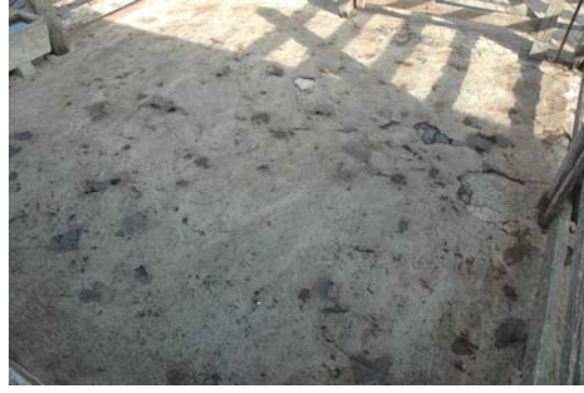
Photo 3.29: Detail of early bluestone paving with introduced concrete slurry over. Note the cracks in the concrete.
