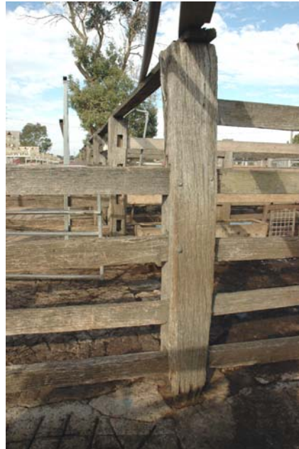
Photo 3.17: Detail of early timber post & rail pen fence. Note the rotting (needling) base of the post and weathered condition of the rails.
