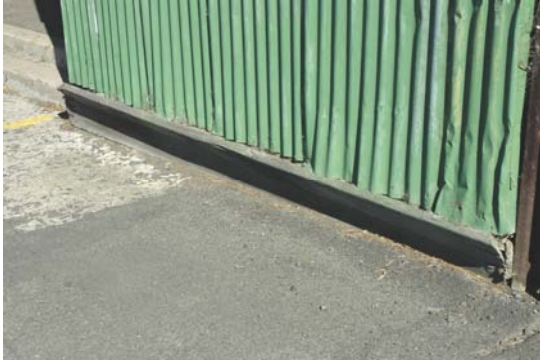
Photo 3.76: Market Offices building, east elevation. Detail of rotted timber baseboard on projecting northern office gable.
