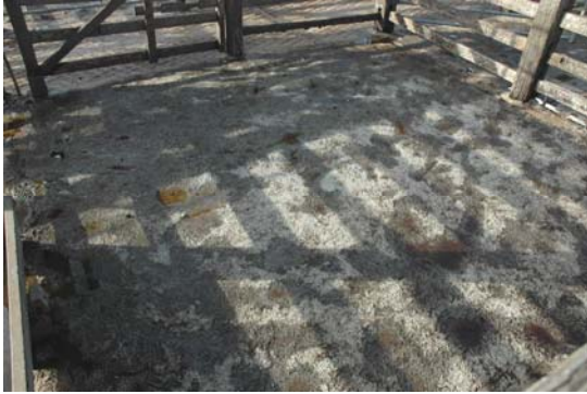
Photo 3.28: Detail of early bluestone paving with introduced concrete slurry over.
