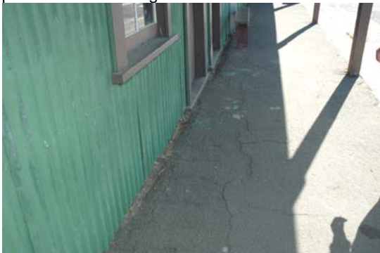
Photo 3.80: Market Offices building, east elevation. Detail of gap between the asphalt verandah floor and the wall base.
