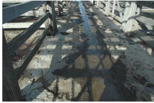
Photo 3.21: Detail of internal way showing invert drain. The concrete slurry over the bluestone has been introduced. Note the cracking and breaking down of the concrete.
