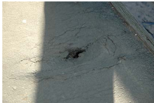
Photo 3.25: Detail of hole in floor of covered walkway, indicating structural breakdown of the timber subfloor structure and timber floor boards.
