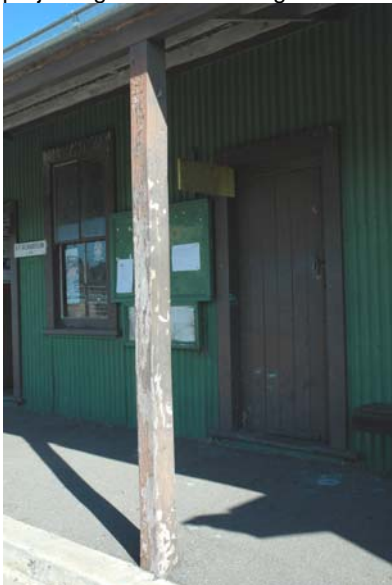
Photo 3.78: Market Offices building, east elevation. Verandah post detail. Note the peeled paint and weathering.
