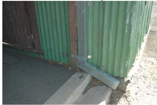
Photo 3.79: Market Offices building, east elevation (south face of projecting northern office gable). Detail of introduced downpipe not connected to sealed drainage.
