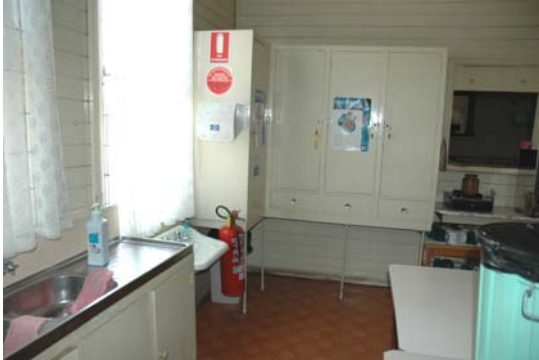
Photo 3.116: Interior, Kitchen, looking north-west. Note substantial slope in floor in the unlevel cupboards.
