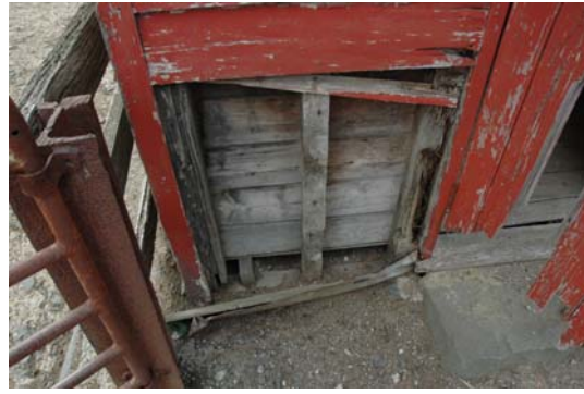
Photo 3.137: Former Caretaker's Cottage, south elevation. Detail of rotted and missing timber weatherboards west of door opening.
