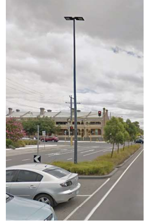
Back to back arrangement installed in Myer Street
