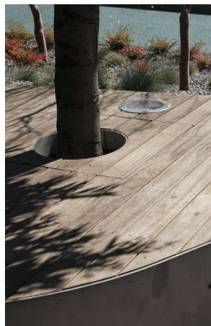
Deck mounted tree uplight in Malop Street
