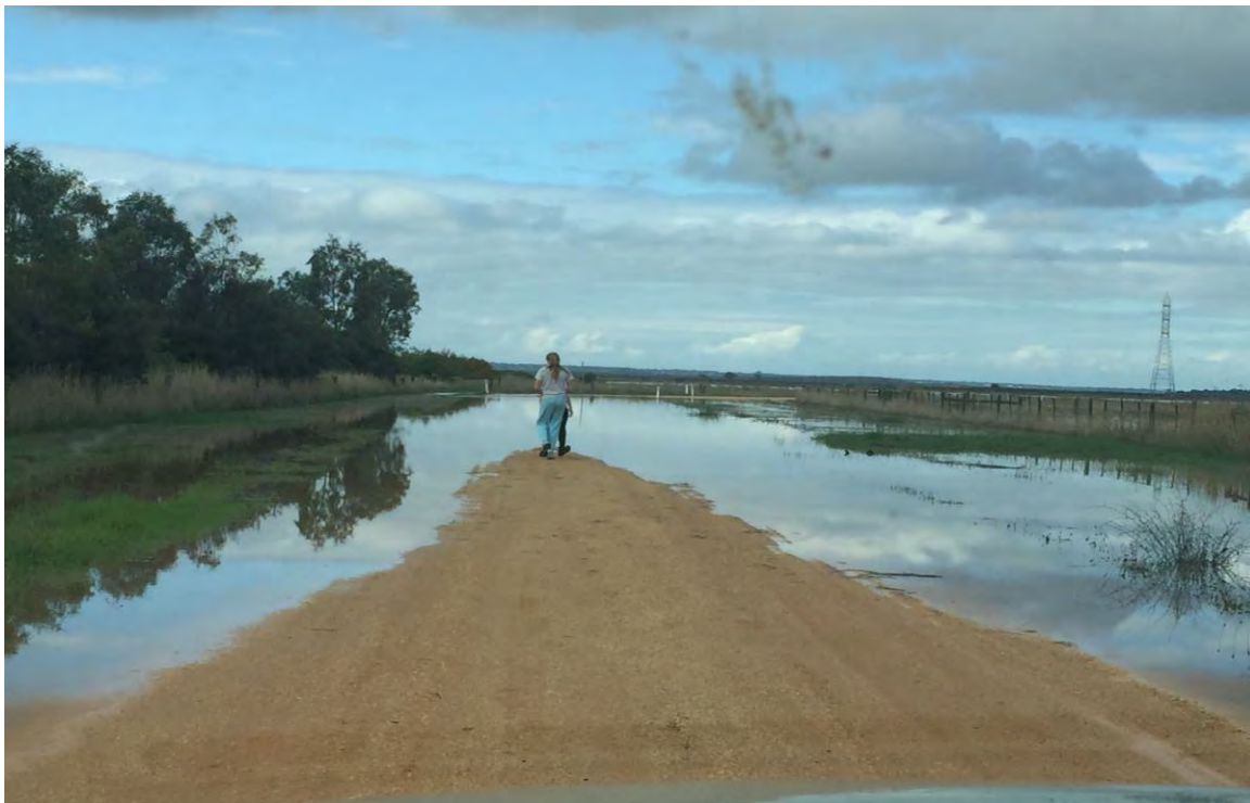
Figure 3 Flooding at Harriott Road 7
