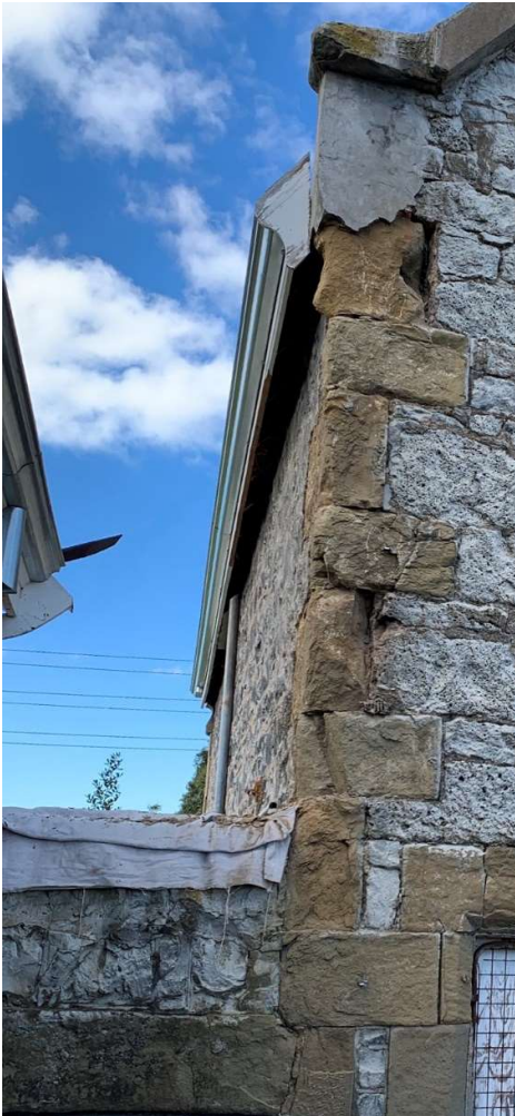
Stone quoinwork, former orphanage, prior to repair. Source: Matt Cartlidge.
