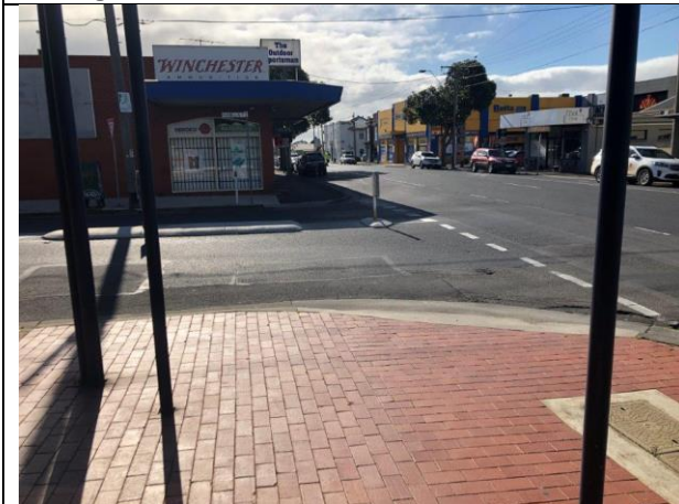
Crossing across Isabella Street, footpath grades to carriageway, gradient approx. 9.5%
