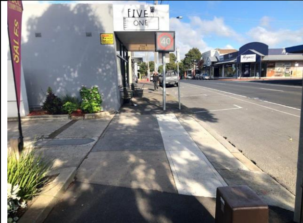
Typical concrete crossover × Crossfalls 4.9%, in excess of 2.5% for concrete
