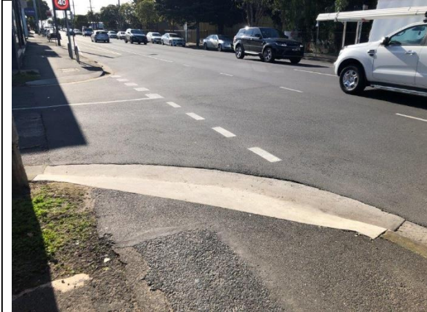
Crossing across Clonard Avenue, footpath grades down to carriageway with gradient approx. 17.3%
