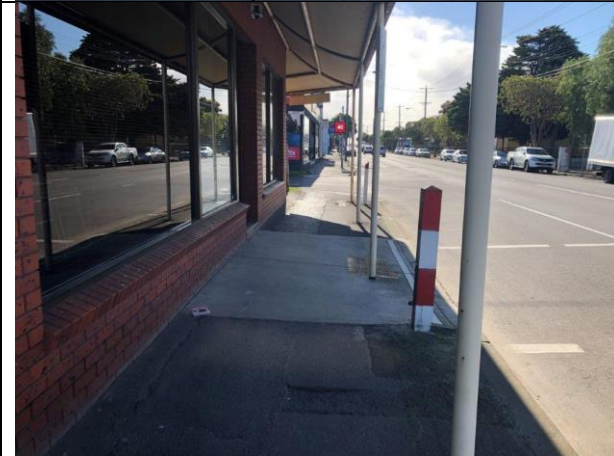
General view – multiple asphalt repairs
