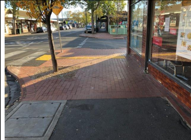
General view × Uneven brick finish adjacent tree
