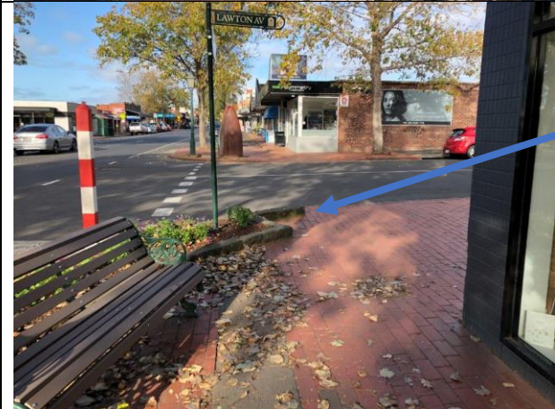
General view × Extension of planter edging creating trip hazard
