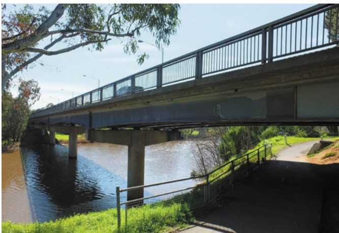
Figure 3.27: Princes Bridge looking north from the south bank of the Barwon River, 2019. Source: David Rowe.
