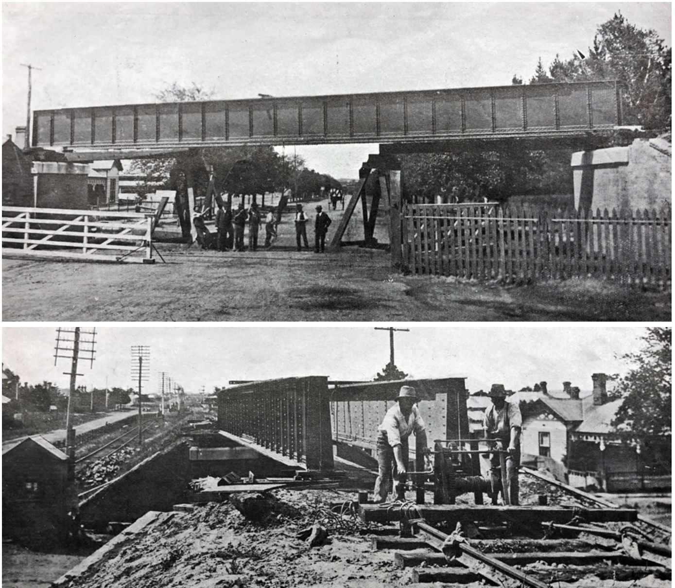
Figure 3.108: Moorabool Street Railway bridge nearing completion, 1912. Source: News of the Week , 12 November 1912, p.14, GRS 2121/3, Geelong Heritage Centre collection.
