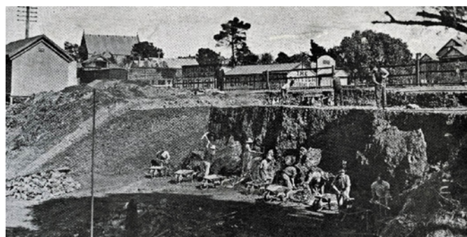
Figure 3.99: Subway under excavation, 1912. Source: News of the Week , 22 August 1912, GRS 2009/01404/029, Geelong Heritage Centre collection.
