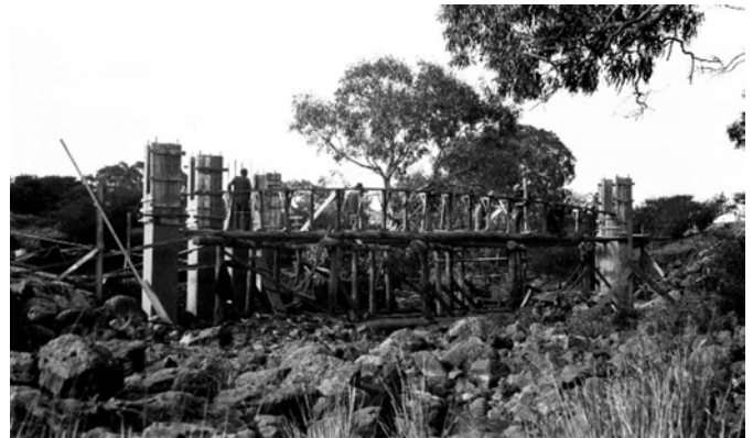
Figure 3.36: Ripley Bridge under construction, photographic collection, Roads Corporation, 1928. Source: VPRS 17684/P3 it 28/00021. Public Record Office Victoria.
