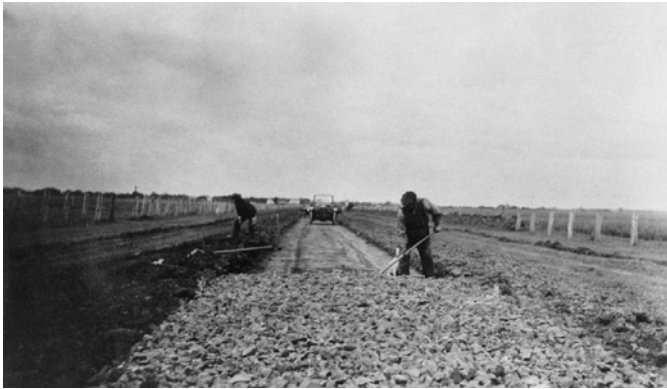
Figure 3.06: Geelong to Melbourne Road under construction, photographic collection, Roads Corporation, 1913. Source: VPRS 17684/P3 item 13/00153 Public Record Office Victoria.
