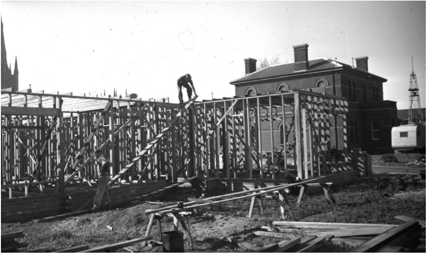
Figure 7.88: Dwelling for the District Engineer of the Country Roads Board under construction next to the old Police Station, McKillop Street, 1947. Source: VPRS 17684/P3 item 45/04448 Public Record Office Victoria.
