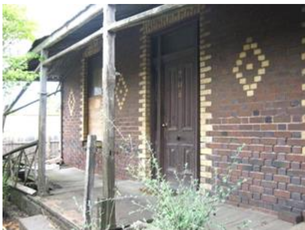
Victorian front verandah in disrepair. Remnant fabric in good condition was retained and used as a basis for reconstruction. Source: Jennifer Bantow.
