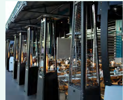
Image 08. Heating devices located within Trading Zone with adequate height clearance to sit within the building awning.
