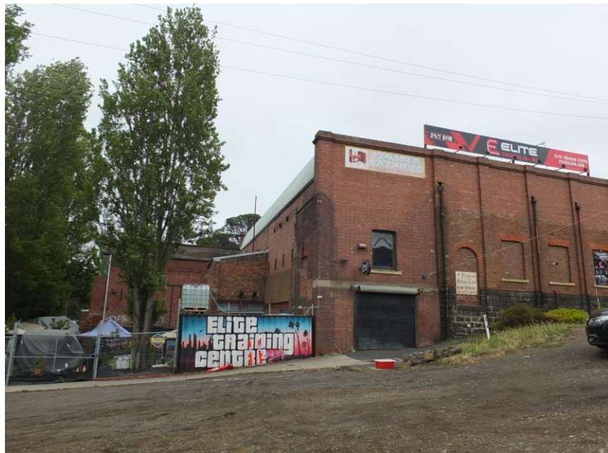
Former Albion Mill, east elevation (south wing and southern portion east elevation of main building), December 2023. Source: David Rowe.
