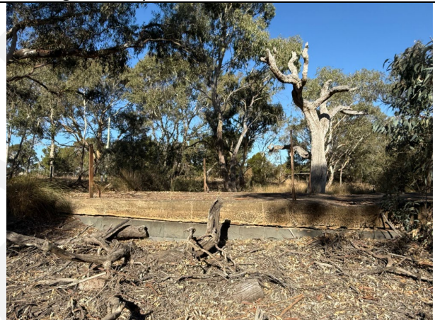
Oblique view of the eastern elevation of the Weir. Source: City of Greater Geelong, February 2025.
