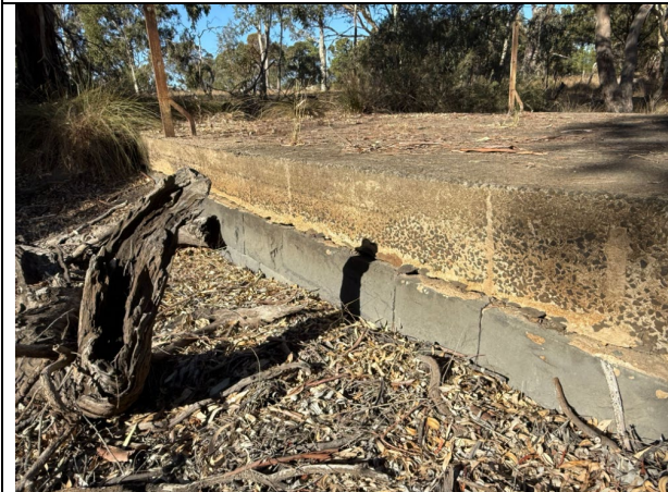
Detail view of the 1930s concrete deck on the weir. Source: City of Greater Geelong, February 2025.
