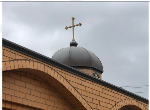
View of the eastern cupola, looking east. Source: City of Greater Geelong, September 2024.
