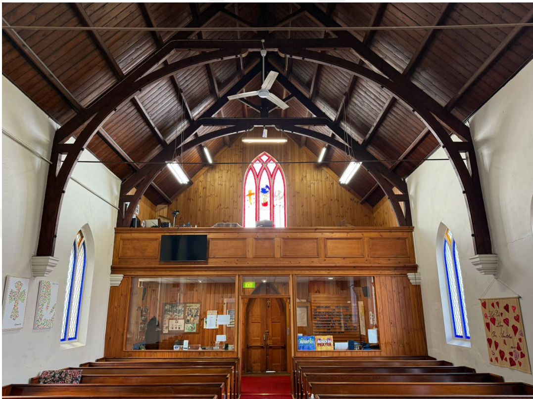
Figure 8. Interior view of St. Paul's Lutheran Church in October 2025. Note: no internal controls are proposed, as such no furnishing or material finishes are proposed for protection. Source: City of Greater Geelong, October 2025.
