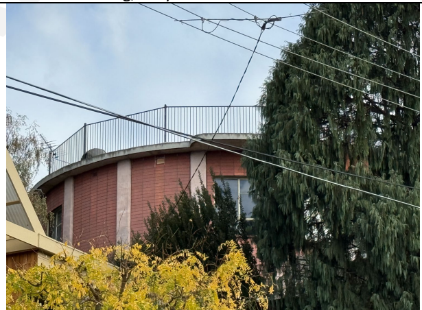
Detail view of the roof showing the railing. Source: City of Greater Geelong, May 2025.
