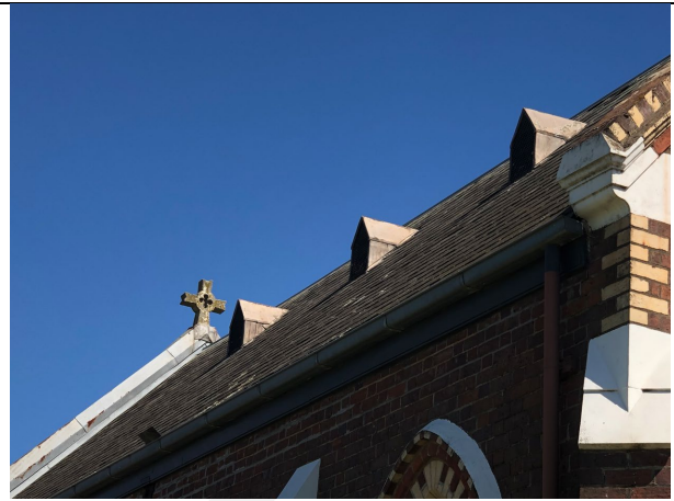
Overview of the dormer roof vents, crucifix and introduced cladding to the rear parapet. Source: City of Greater Geelong, November 2024.
