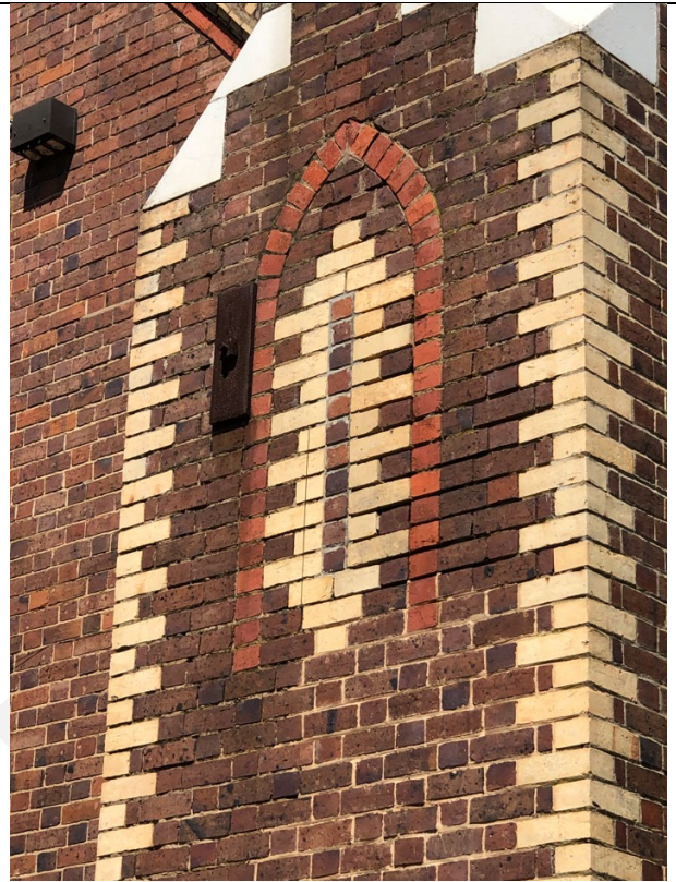
Detail view of filled in archers slit. Source: City of Greater Geelong, November 2024.
