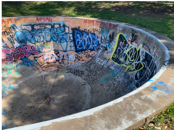
Detail view of the third, and most challenging, hemispherical bowl. Source: City of Greater Geelong, February 2025
