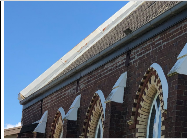
Detail view of repointing work and steel-ties. Source: City of Greater Geelong, November 2024.
