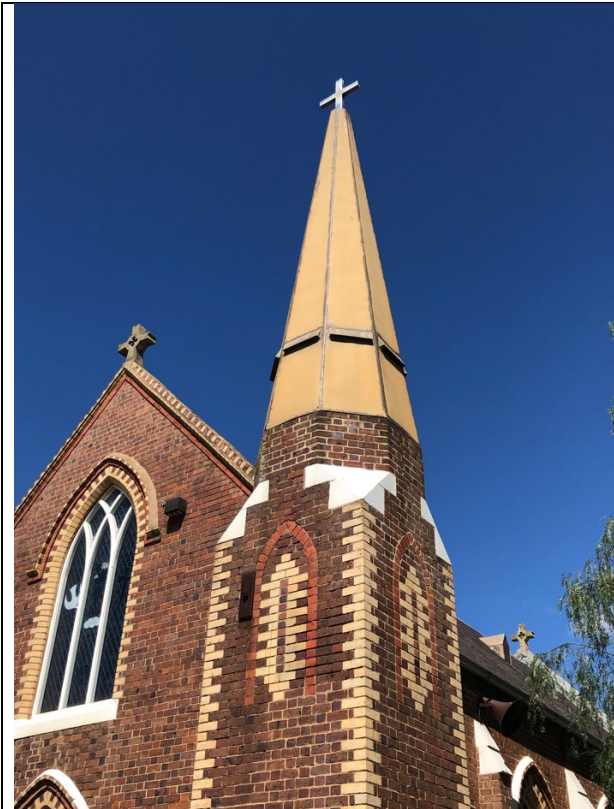
Oblique overview of the altered tower, looking southwest. Source: City of Greater Geelong, November 2024.
