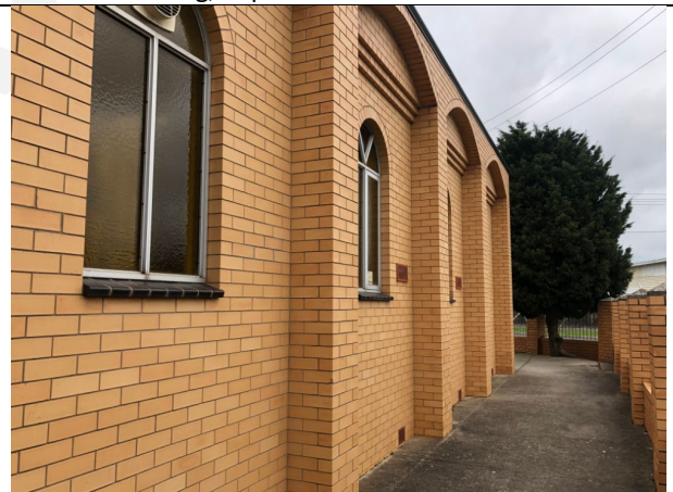
Oblique view of the northern elevation of the Church. Source: City of Greater Geelong, September 2024.
