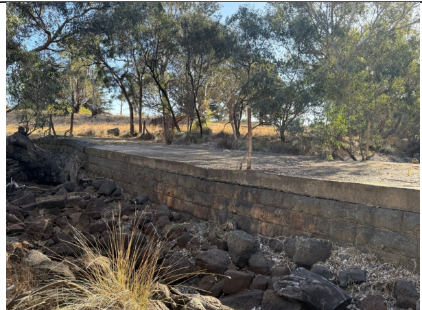
Oblique view of the Ripley Weir looking southeast from the northwestern embankment. Source: City of Greater Geelong, February 2025.
