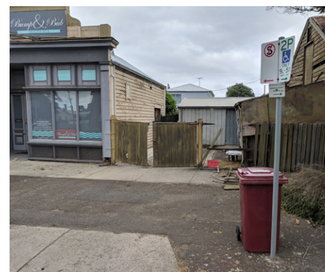
Shop, 164 Bellerine, Street, 2018, showing signs of dilapidation.
